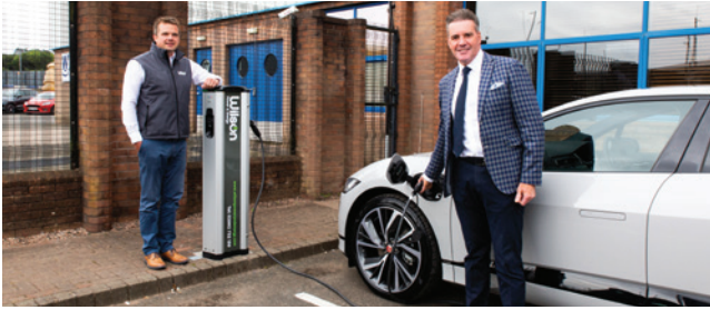
Peter Johnston, Wilsons Auctions Group Operations Director (right) with Andrew Wilson, Managing Director of Wilson Power and Energy Ltd who installed the new EV chargers at Wilsons Auctions' premises.
